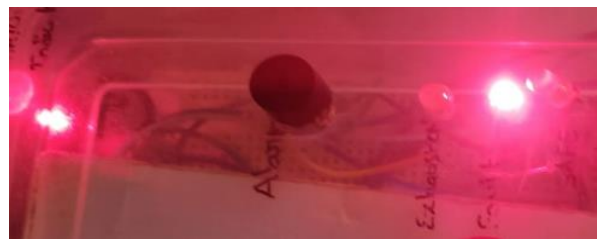
Fig. 16. Fault Indication at local BMU
